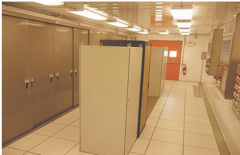
Figura 7: Vista Interna 2 Remote Instrument Enclosure (RIE).
