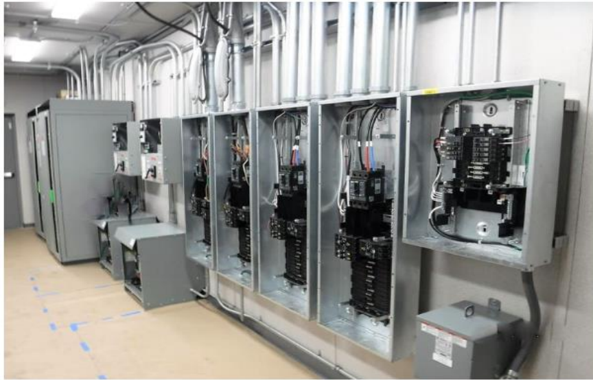
Figura 6: Vista Interna 1 Remote Instrument Enclosure (RIE).
