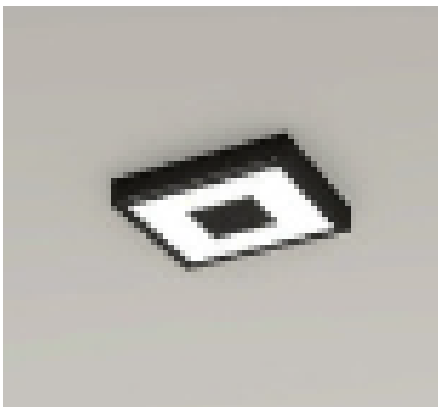
Figura 35 Luminaria led interna
