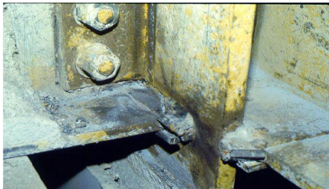
Widespread failure of welded flange - bolted web moment connections
