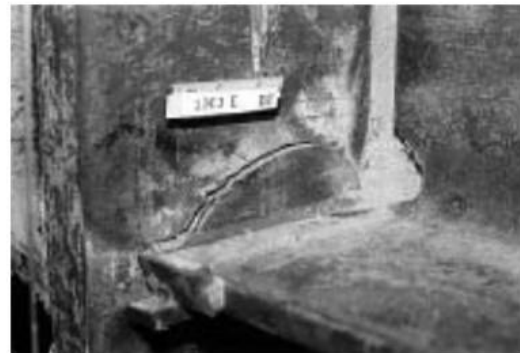
b. Column Flange "Divot" Fracture
