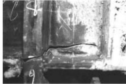
a. Fracture Progresses into Column Web
